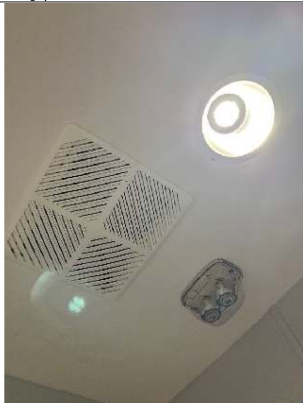
Photograph 7: Lighting and exhaust fan at New Shower 3
