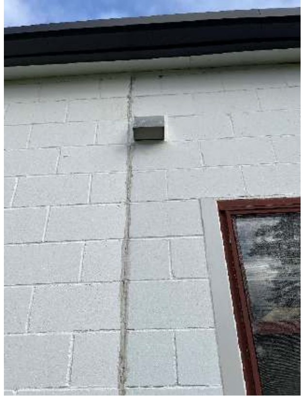
Photograph 10: Exhaust Vent Cover
