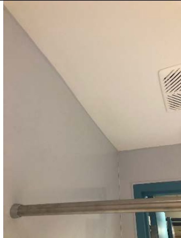
Photograph 13: Correction of deficient painting (photo by M Builds)
