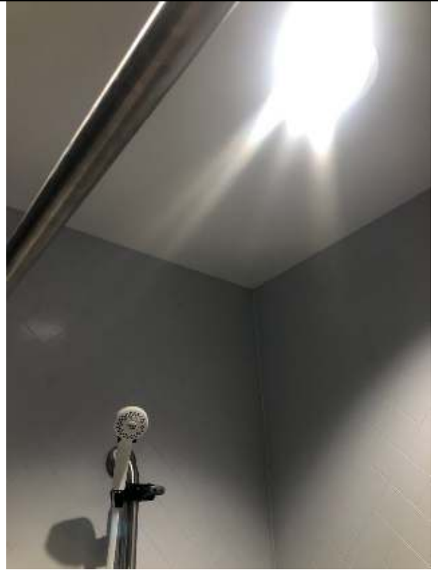
Photograph 14: Correction of deficient painting (photo by M Builds)
