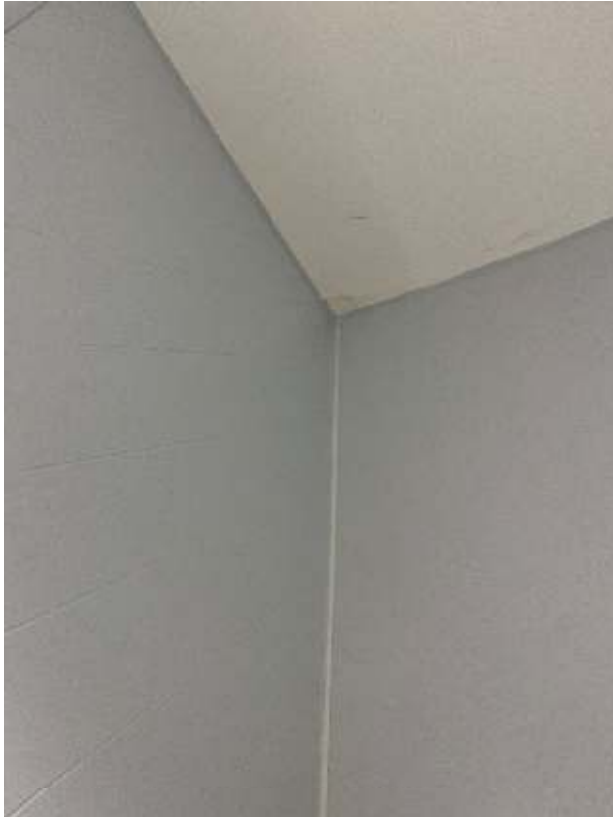
Photograph 11: Deficient painting at perimeter of New Shower 3
