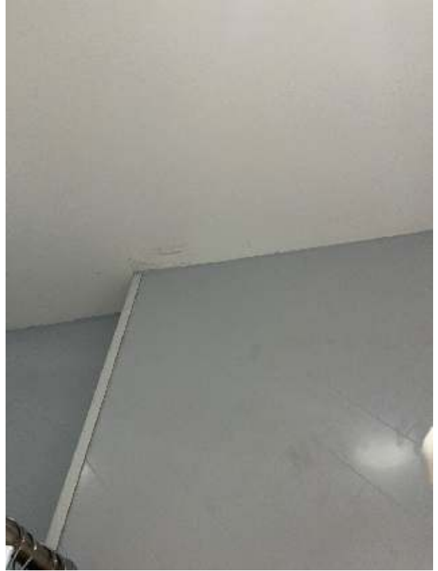
Photograph 12: Deficient painting at perimeter of New Shower 3
