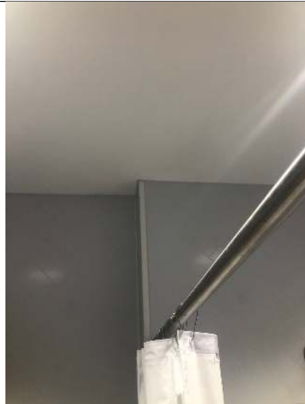
Photograph 15: Correction of deficient painting (photo by M Builds)
